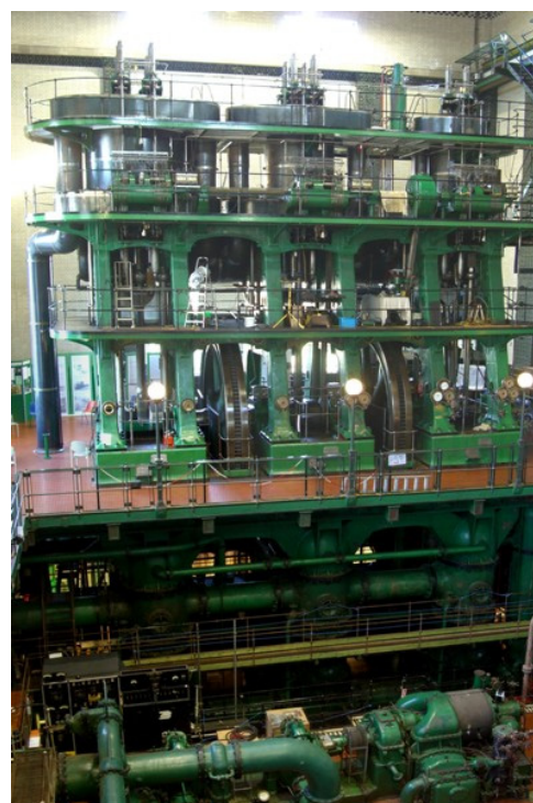
No.6 Triple-Expansion Steam Pumping Engine
