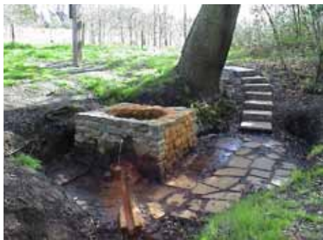
Photos - Rebuilding the stonework around the newly fitted grille; The finished project with steps to reach it safely
